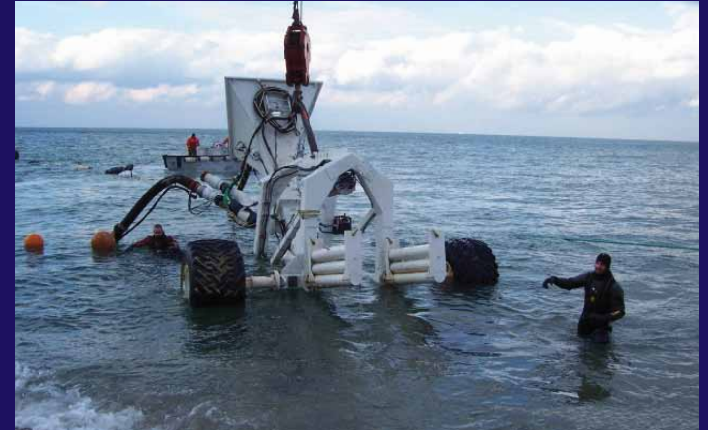
As the plow travels along the seabed, it liquefies the soil ahead of the plow using water jets on the plow blade. The cable passes through the hollow plow blade and is buried approximately 6 feet below the seabed. The temporarily liquefied area almost immediately fills back in as the sediment naturally resettles.
