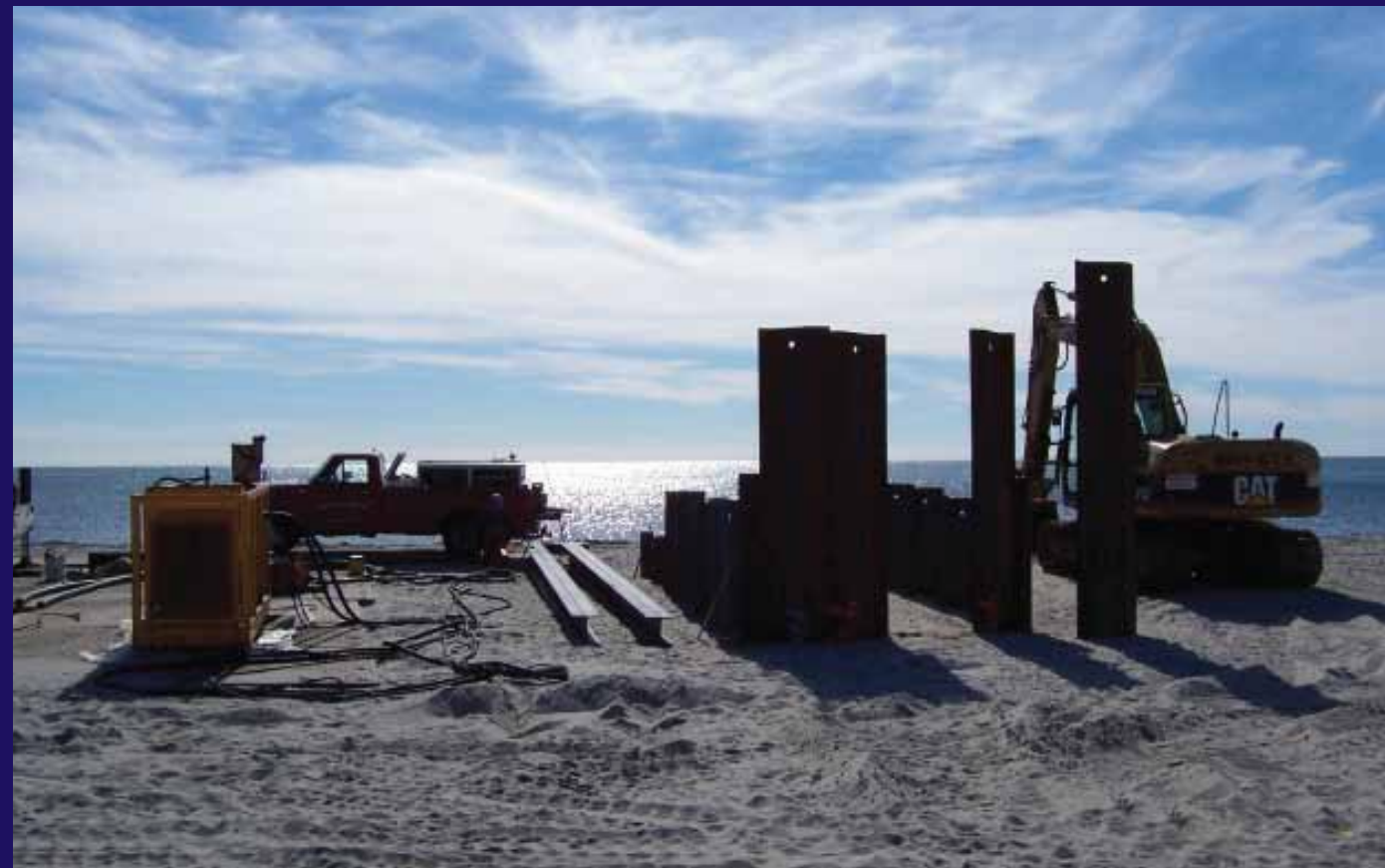
Creation of temporary cofferdam (sheet pile supported excavation) to bring submarine cable ashore.
