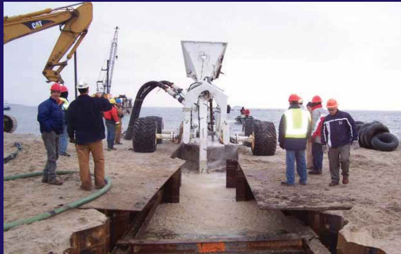
Submarine cable is fed through the plow, which will enter the water and travel along the seabed until making landfall on the opposite side of the water crossing.
